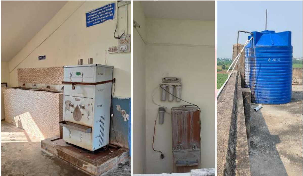
Drinking water facility, Water storing Tanks
