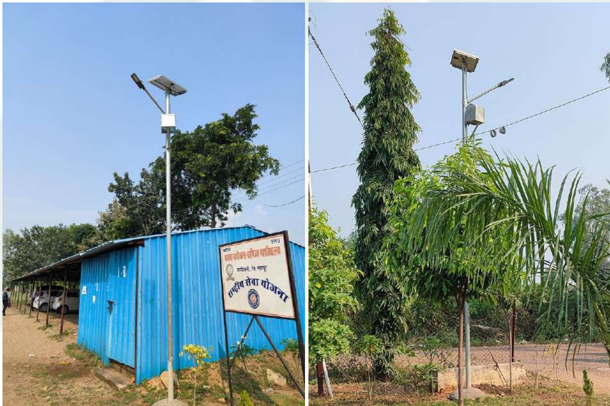
Generator, battery, photocells installed in the college
